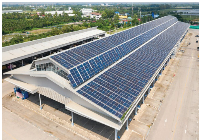
Figure 18: Rooftop solar PV system
