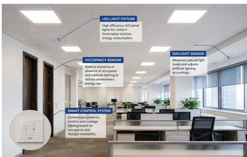
Figure 2 LED Lights with Smart Control System
